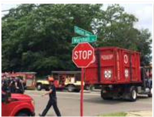
Crews searched for several hours Wednesday before they located the buried body of James Rogers, a worker who had a trench collapse on him in Washington Twp. NICK BLIZZARD/STAFF
